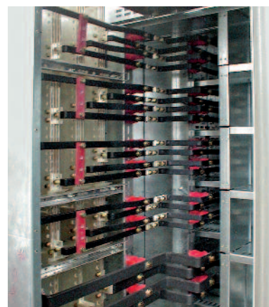
Derivazioni tra calate e interruttori Connections between secondary busbars and circuit breakers
